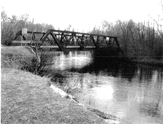
Figure 2: Former County Road 497 Bridge over the Sturgeon River, looking upstream. The Bridge was removed in 2006 but the concrete abutments were left in place. The proposed replacement bridge would be of similar construction (steel pony-truss bridge with concrete deck) but be 20 feet longer and 10 feet wider.
