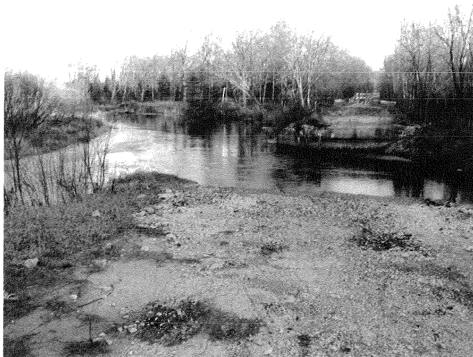
Figure 5: Constriction of the Sturgeon River by bridge abutments installed circa 1917. Bank scour upstream of bridge can be seen at left middle ground and on the opposite side of the river, upstream of bridge abutment. Flow is from left to right.
