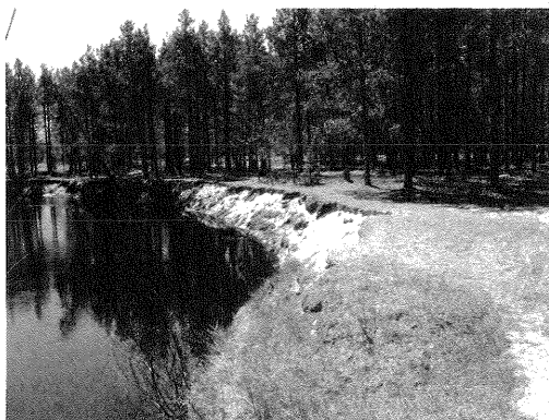
Figure 5: First Meander Bend immediately downstream of the proposed project site. Inadequate span of original structure likely contributed to bank erosion of the deep, droughty, infertile sands adjacent to the river.
