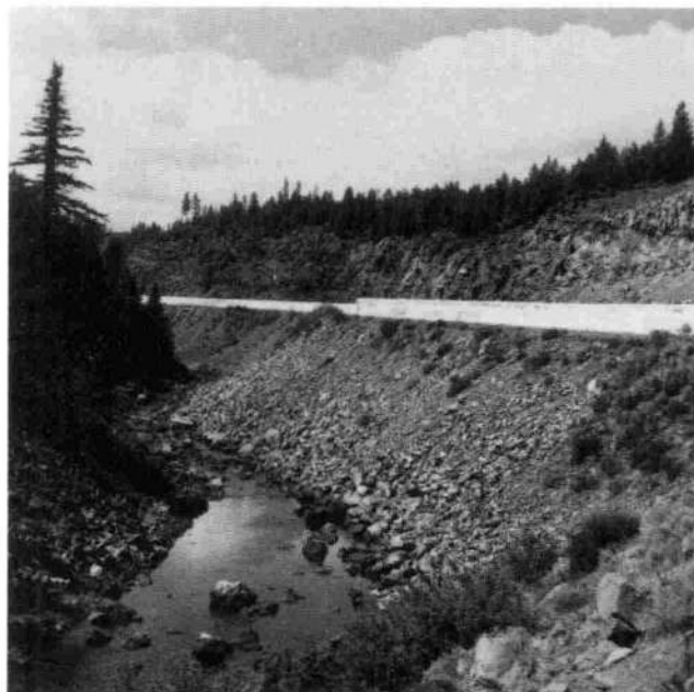
Above-ground flume and shoreline modification in segment 1.
